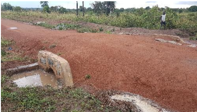
Ch. 5+900: Chocked culvert crossing due to lack of RMM
