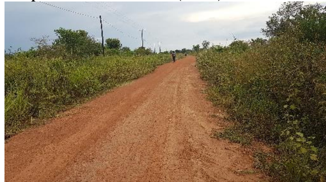
Ch. 1+200: Lack of routine manual maintenance
