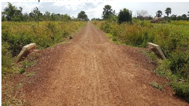
7+300: Culvert installation with inadequate backfill
