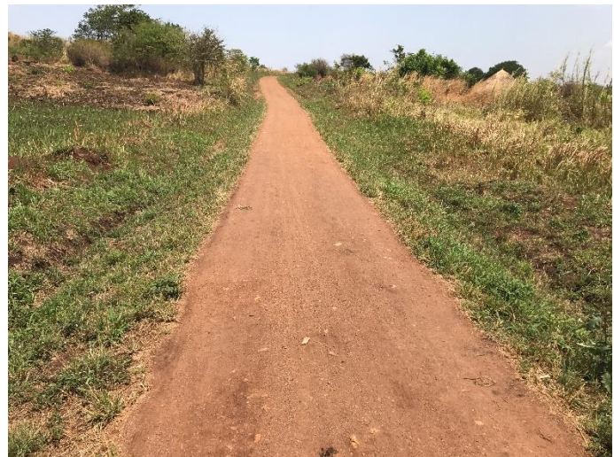
Ch. 6+100: Narrow carriageway
