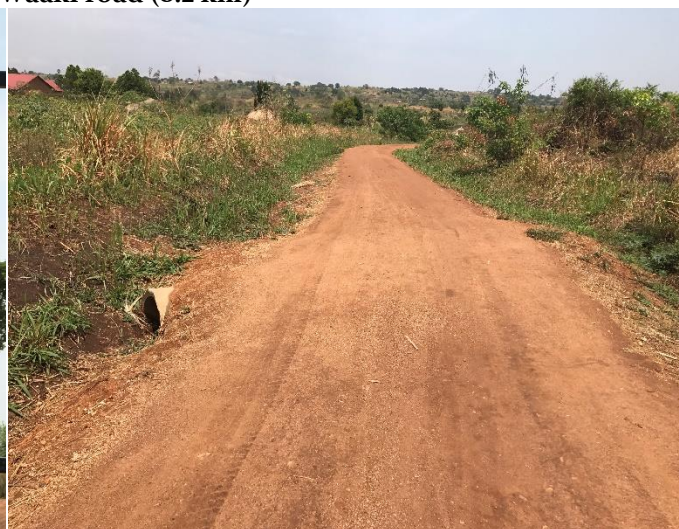
Ch. 1+100: Culvert installation with loosely compacted backfill
