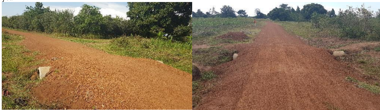
Ch. 0+600: Culvert installations lacking end structures Ch. 2+600: Culvert installations lacking end structures
