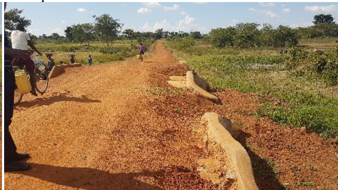
Ch. 6+200: Exposed concrete culvert pipes due to inadequate backfill material
