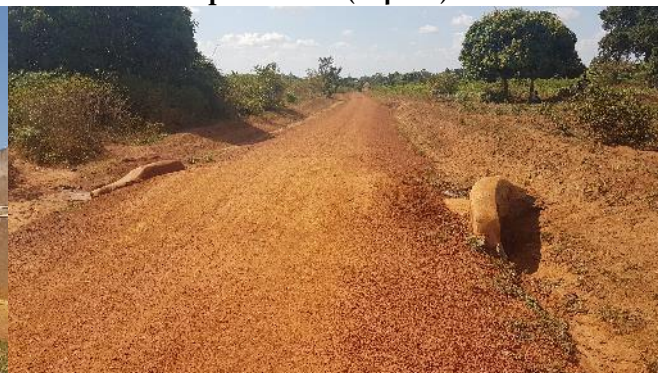
Ch. 0+200: Exposed concrete culvert pipe due to inadequate backfill material
