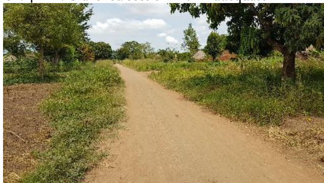
Ch. 20+600: Lack of RMM
