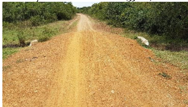
Ch. 16+600: Poorly compacted culvert backfill
