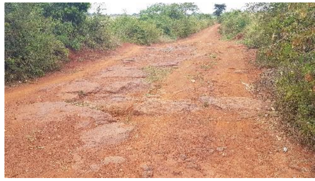
Ch. 31+900: Rock outcrop requiring gravel filling
