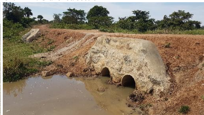
Ch. 8+200: Multiple culvert installations in swamp crossing. Embankments require protection by installation of gabion walls
