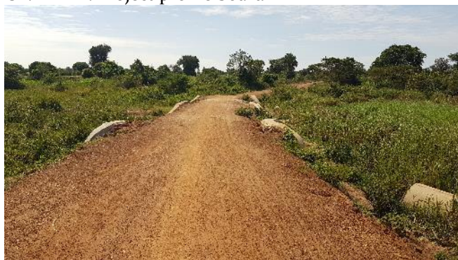
Ch. 4+500: Multiple culvert installations in swamp crossing. More fill material is required
